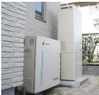
Home use fuel cells are installed in all 14 detached houses
