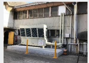
The new chiller
