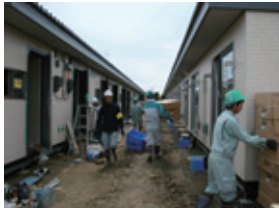
Construction personnel worked from early morning until late at night, including weekends.
