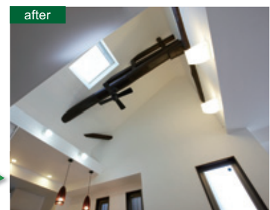
The large ceiling beam is effectively used in the renovation of the room
