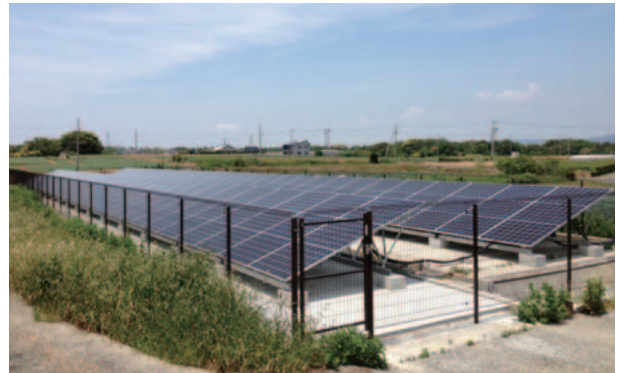
A mid-scale solar project makes effective use of idle land
