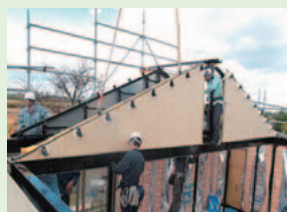
Installing a precut piece of plasterboard as boundary wall for an attic
