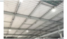
Switch to LED ceiling lighting at a panel factory
