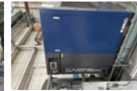
Upgraded to high-efficiency compressors
