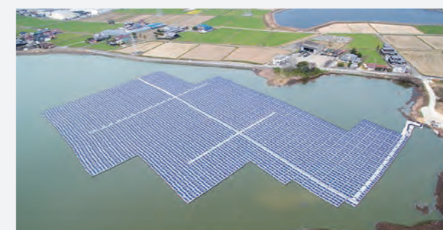
Floating solar system
