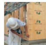
Technician training is an important area of focus
