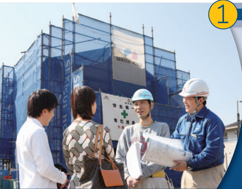
All workers involved in a homebuilding project act from the customer's perspective
