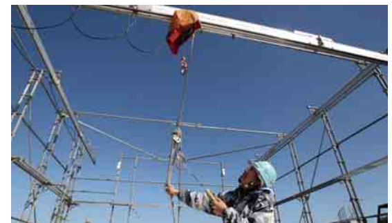
We use our proprietary “girder crane” system on the construction site. We conduct frame construction and exterior work using an overhead crane that is temporarily installed on the upper part of scaffolding.
