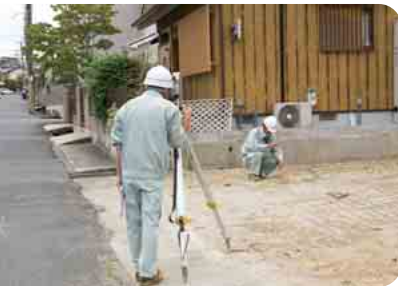
In a site survey, we check the exact gas and water pipe locations.
