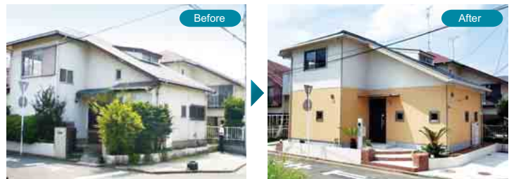
Structural, interior and exterior components, room layout and fixtures are renovated to the latest standards by our proprietary remodeling technology.
