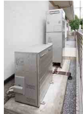
Fuel cell system for residential use
