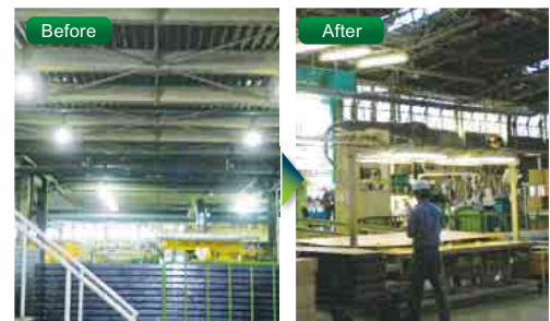
Mercury lamps for general lighting were replaced with fluorescent lamps for close lighting.
